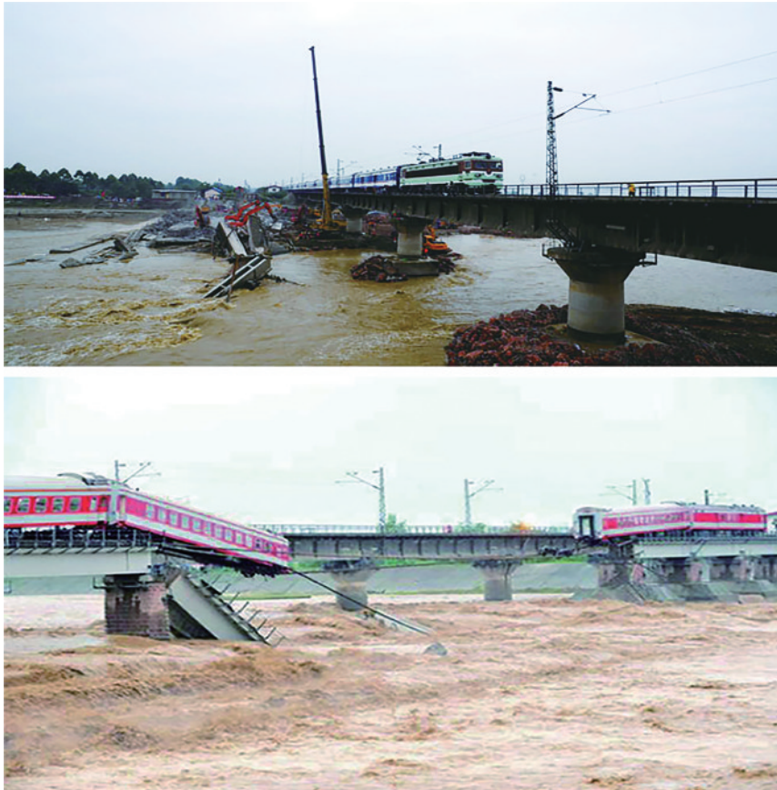
Fig. 1 Shiting River Bridge on Baoji-Chengdu Railway having been destroyed by floods
