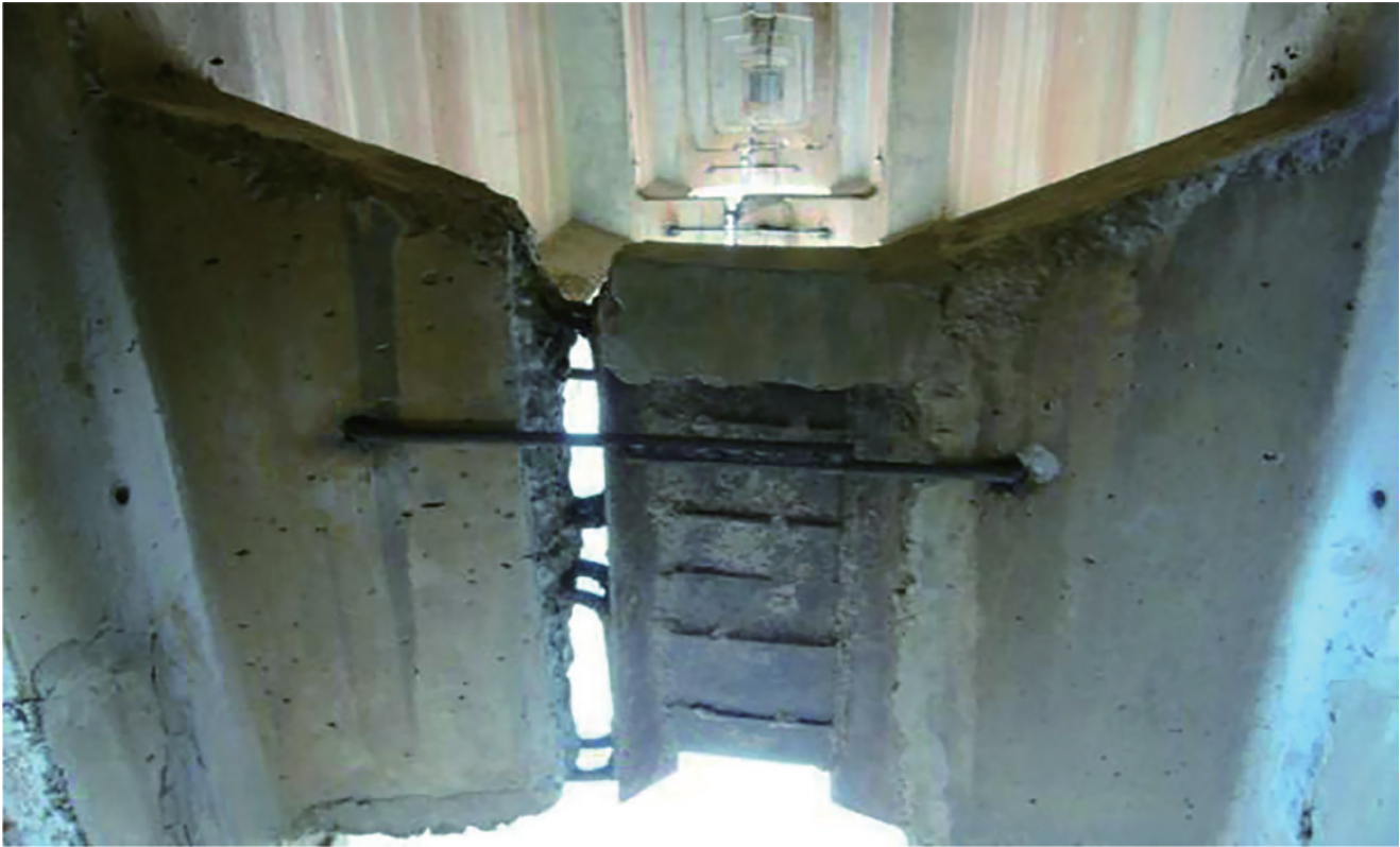
Fig. 12 Deterioration phenomenon of simply-supported T-beam on mixed passenger-freight railway
