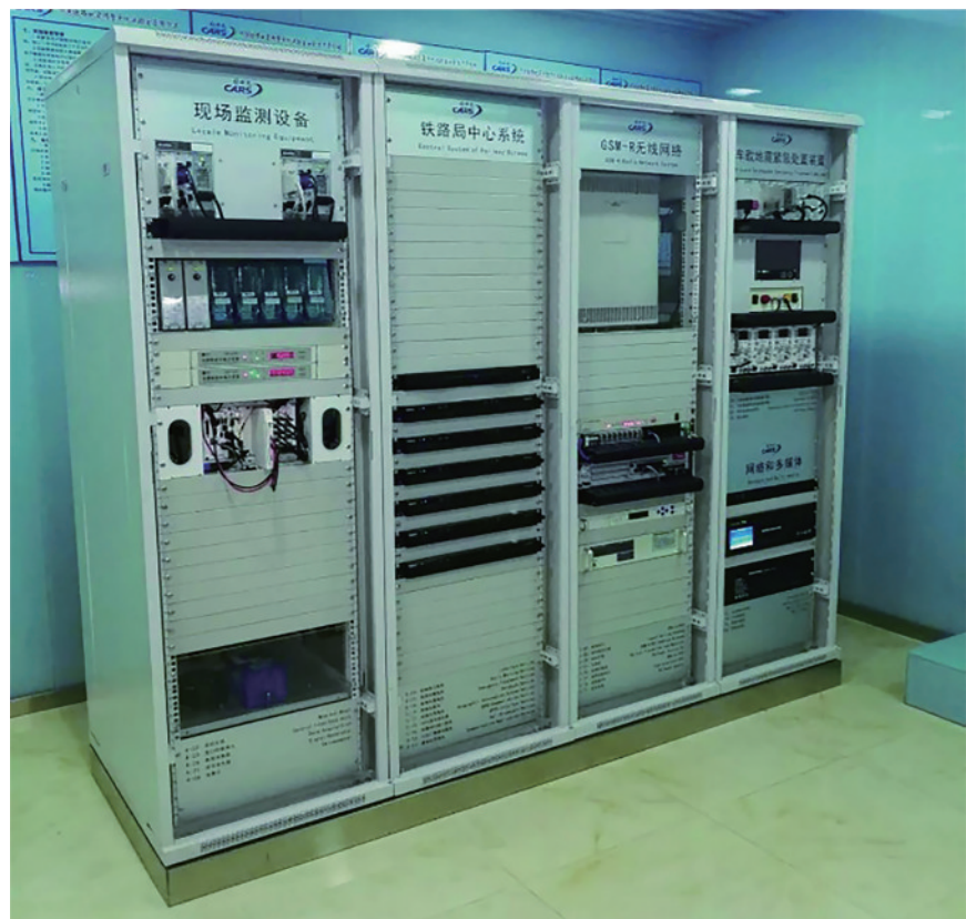
Fig. 11 HSR earthquake early-warning system
